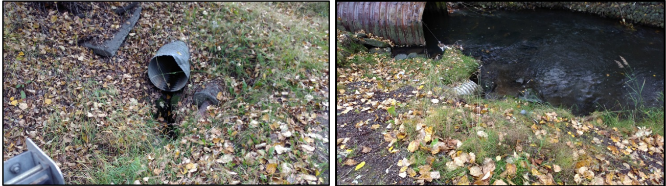
Figure 2. SWM07 Outfall Configuration.
